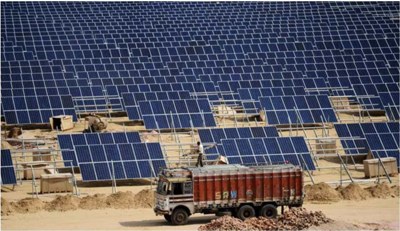
Indian engineer positions solar panels at the construction of the Roha Dyechem solar plant at Bhadla in Rajasthan, India. Photo by Money Sharma/AFP via Getty Images.
